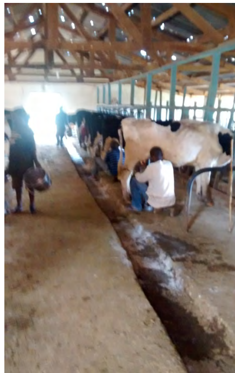
Deteriorated floor, rafters, and roof
