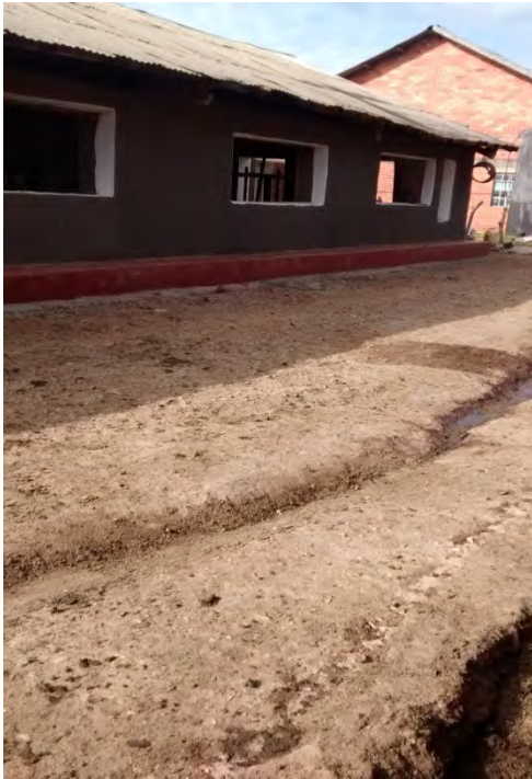
Milk barn - Exterior walls upgraded - Eroded walkway - and deteriorated roof
